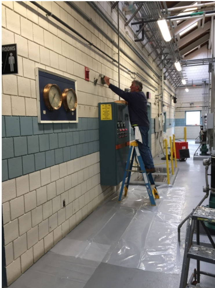
Beautifying the chemical feed room.
