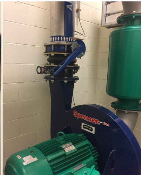
Cocheco Well Blower #2
