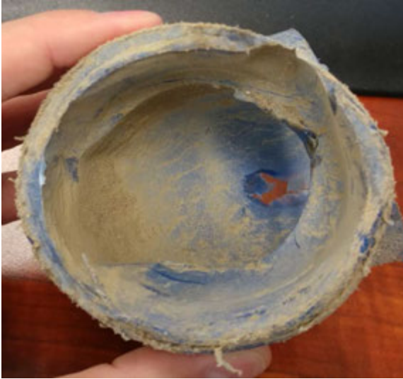
Eroded/failed air scour line
