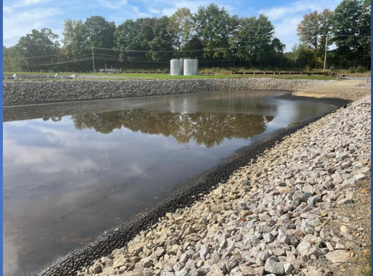
Lagoon B Buildup of 4.75 Feet of Sludge and Water (September 2022)
